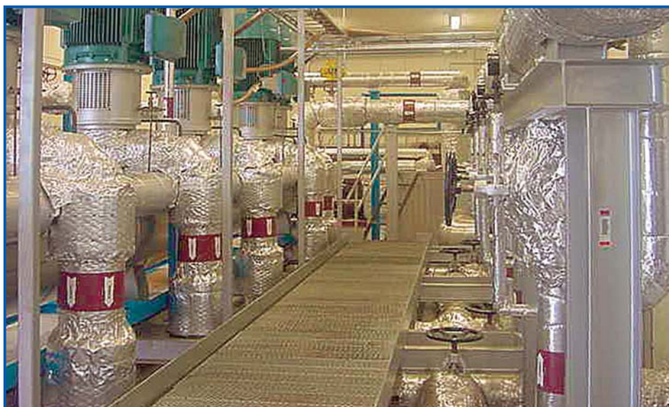
View to Trelleborg Rubore's clean pump room of the Hydro-Dyn press for the production of rubber steel compound material
