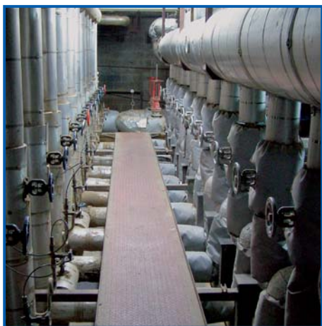
“Old fashioned – but kept clean and still working properly”. High pressure pumps with tubing of Flakeboard’s continuous particle board press
